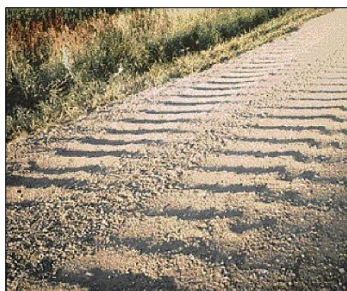
Corrugations. The 4 primary causes of corrugations in gravel roads: (1) driving too fast, hard braking), (2) lack of moisture in the surface gravel, (3) poor quality gravel, and (4) tire slippage on steep grades.
