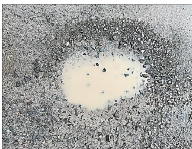
Potholes. Causes include excess water and traffic. The combination removes fine materials from the surface gravel.
